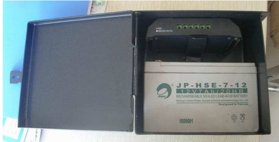
Figure 3. Battery and Charge Controller in Box
